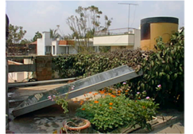
Solar Water Heater
